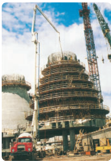
Figure 4 An apparatus that looks like the Canadarm was used to pour concrete.
