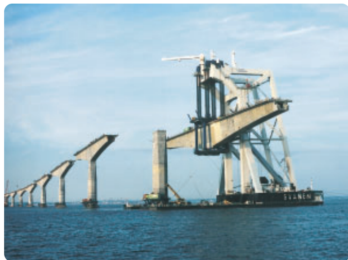
Figure 2 The Svanen , a barge with a floating crane, was used to carry and install the bridge sectors.
